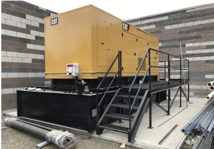
Figure 16: Typical Stationary Back-Up Diesel Generator with Belly Tank Fuel Storage
